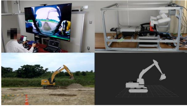
Fig. 8. Photograph and schematic of the teleoperation experiment using a backhoe operated by the proposed system. Operator (upper left), relay device (upper right), actual backhoe (lower left), and estimated posture of the backhoe (lower right).
