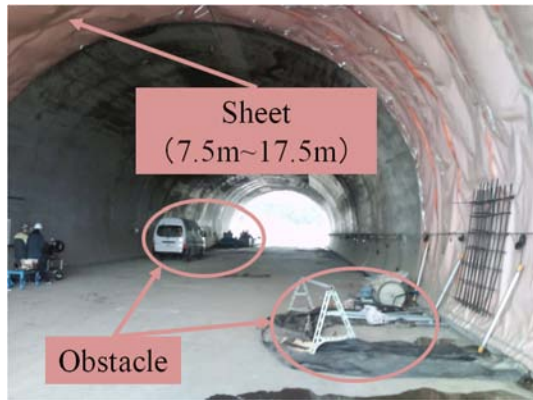
Fig.11 Obstacles in tunnel
